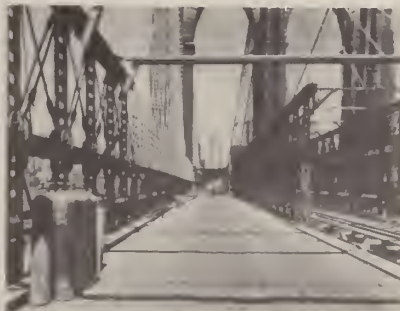
The raised outer truss was braced with struts (horizontal beam) connecting to the inner truss.
